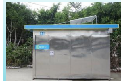
Public Toilet of Pioneers Environmental Technology JSC
